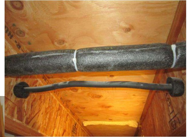
Supply and return water delivered through 1/4 " mini-split line set tubing. Open loop system for system simplicity. All water run at 120F, controlled BTU output through restricted flow to hot water coil
