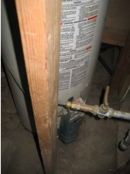
12 year old back drafting natural draft water heater vented to the attic
