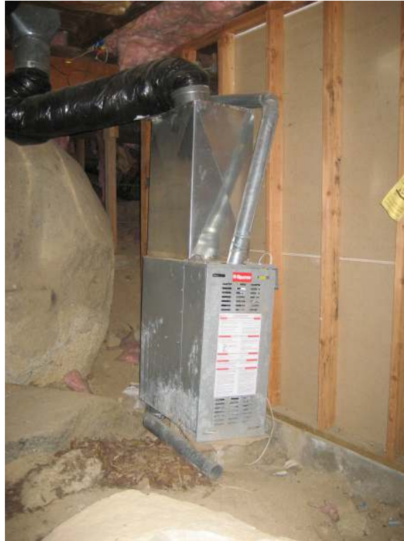
15 year old natural draft furnace installed with no return air duct, return siting directly on dirt, and a single supply duct with booster fan.
