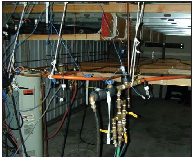
Figure 4. Test Rig for Uninsulated PEX-Al-PEX
